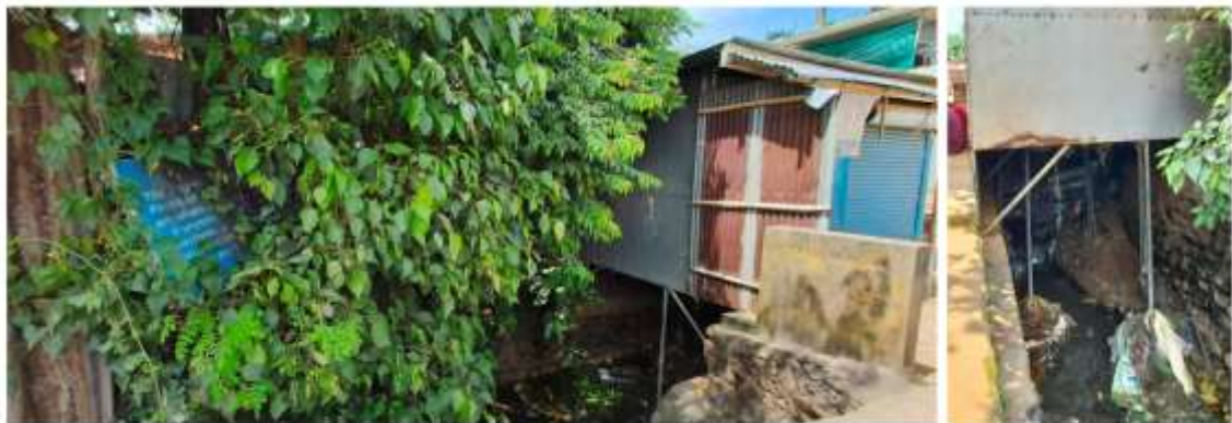
Figure 15: Images showing encroachment on the drainages of Dimapur
