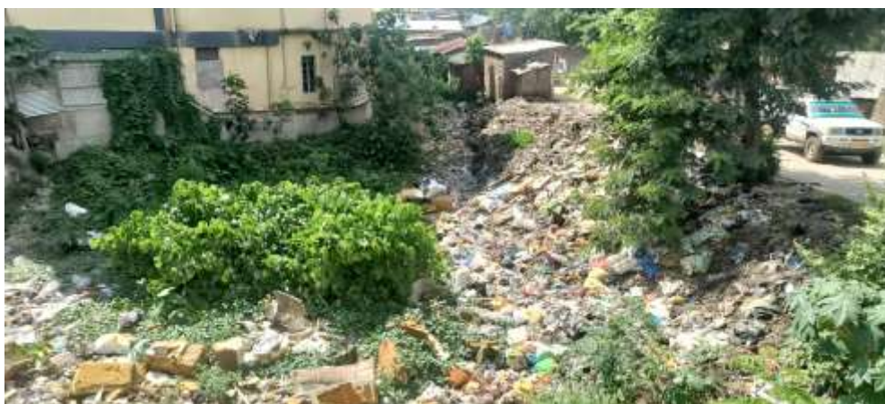
Figure 18: One good example of where slope stabilization can be done
