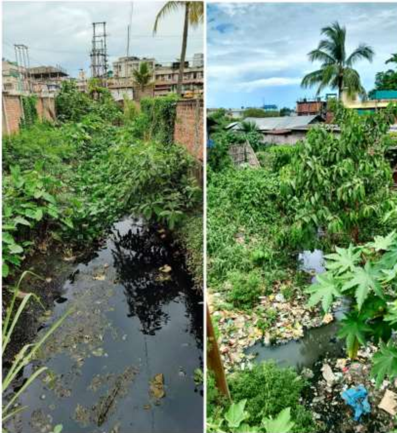
Figure 14: Images showing the growth of vegetation in the drainages of Dimapur
