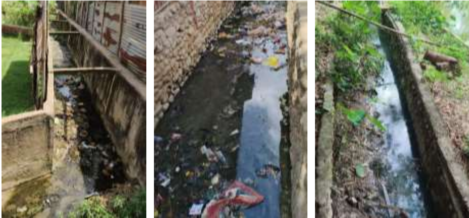
Figure 20: Examples of drains that need covering to prevent garbage dumping
