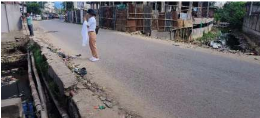
Figure 19; Existing culvert in the Walford area that has to be improved because it is extremely close to the road surface
